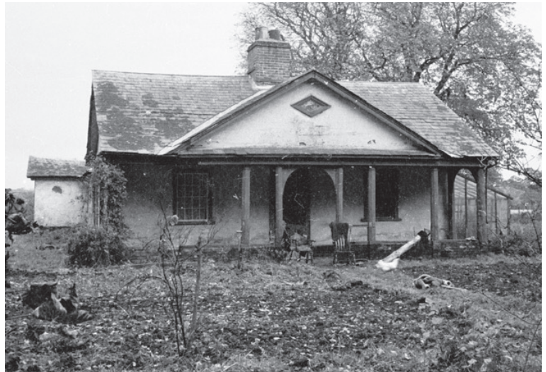
The north side of Wood Lodge, facing towards the present main Ipswich to Hadleigh road (A 1071)
