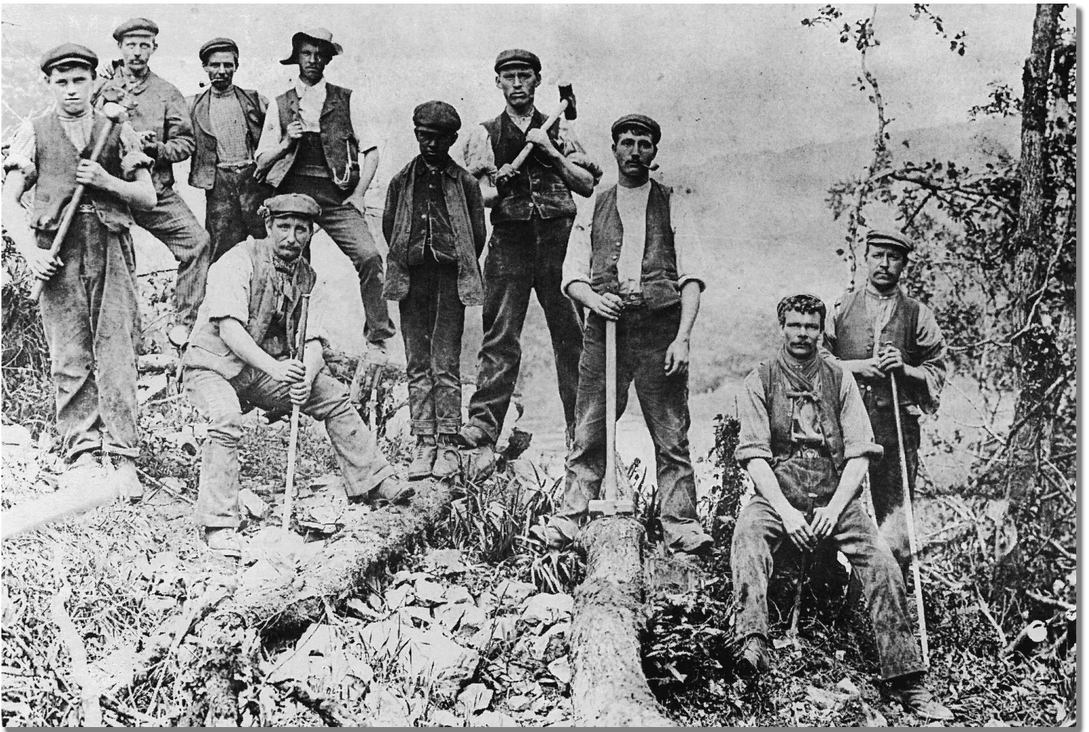
Navvies laying the railway track at Treffgarne Gorge, Pembrokeshire. Western Telegraph / People's Collection Wales / Creative Archive Licence , https://www.peoplescollection.wales/items/2062606#?xywh=500%2C49%2C1303%2C928 .
